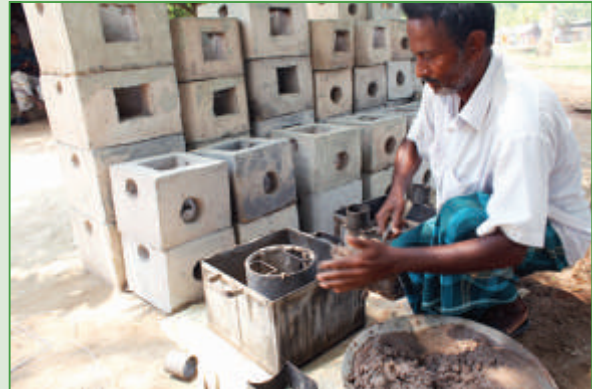
Since its inception, the SED Program has disseminated over 400,000 domestic stoves and over 3000 commercial stoves. Over 2000 people are earning their livelihood through improved stove installation and maintenance.
